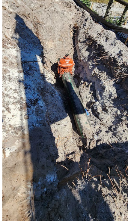
2 - Gate Valve at STA 149+50
