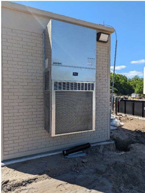
2 – Electrical Building A/C Unit
