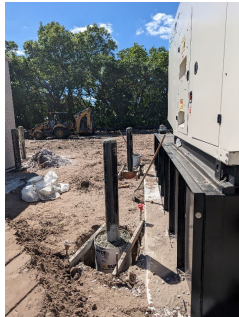
3 - Bollards at Electrical Building
