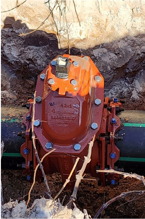
1 – Gate Valve at STA 144+50
