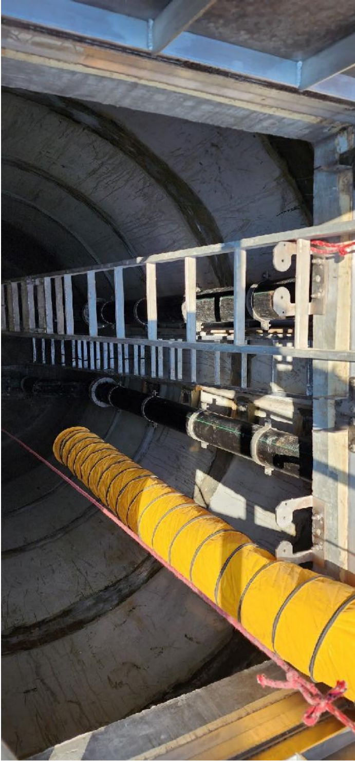
3 – Pump Discharge Risers in Wet Well
