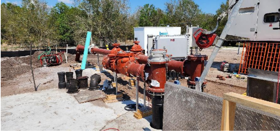
1 - Above-ground Piping Assembly
