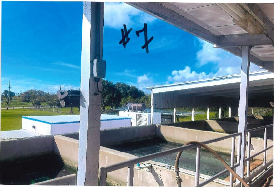
Scope of Work: Photo #7
