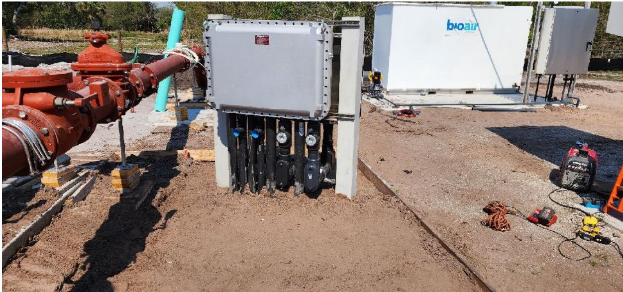
2 - Discharge Piping, Junction Box
