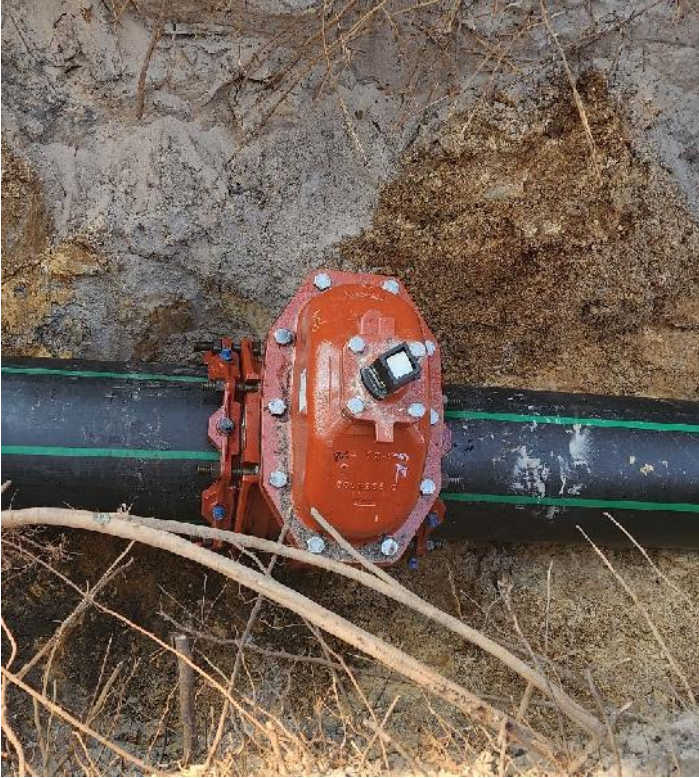
2 – Gate Valve at STA 161
